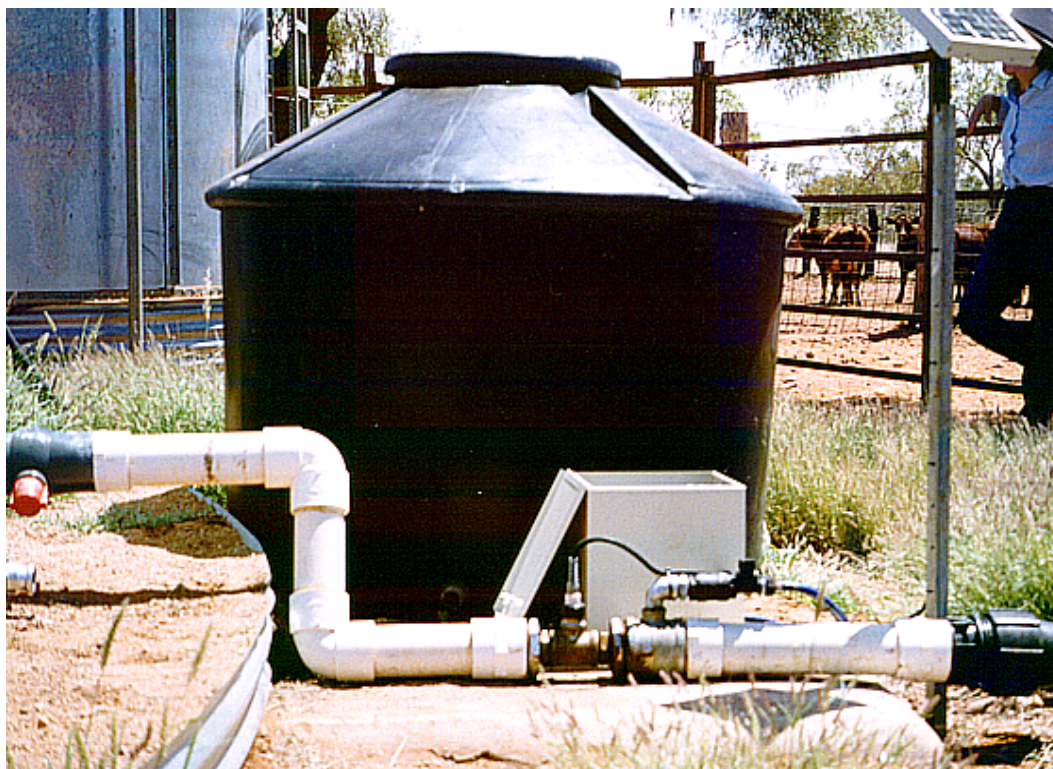
Figure 1. Water medication unit - on property installation
