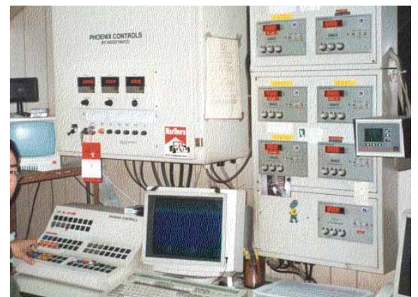
Batch Controllers interfaced in a Computer/PLC batch plant.
