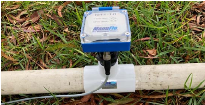
RPFS-LOD installed on a 50mm PVC pressure pipe line using PVC50 adaptors.
